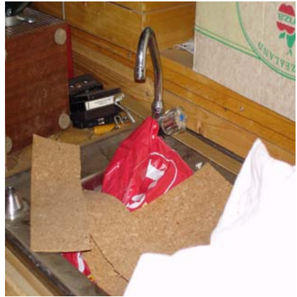
There are serious doubts about drinking water coming out of this point of supply of the bar sink in a forgotten cellar bar (Figure: J. Scheele)
