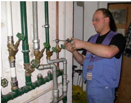
Even if everything was built according to the applicable rules - there is no right of continuance for drinking water systems (Figure: J. Scheele)
