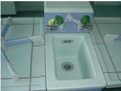
Hose connections in chemical laboratories must be protected with a hose or system separator
