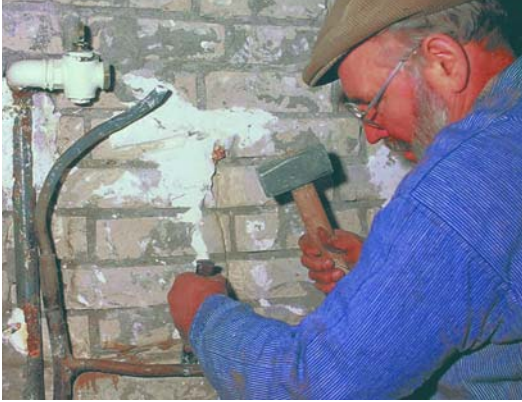
Lead pipes should be removed from drinking water systems as quickly as possible (Figure: SBZ)
