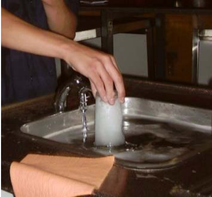
The bottom rinsing pipe of a glass washing facility may only be supplied with drinking water via a free outlet
