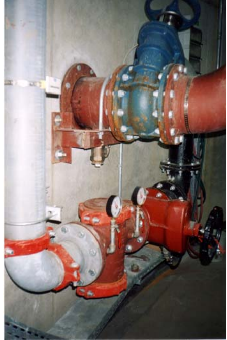
Fire-extinguishing pipes frequently require a nominal width that does not permit the pipes to be flushed sufficiently by the normal water consumption of a house (Figure: J. Scheele)
