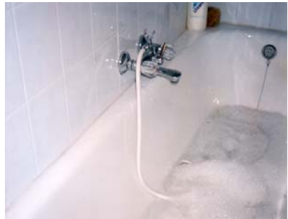
Vulnerable points of supply are, for example, points where the drinking water outlet can be below the level of the non-drinking water
