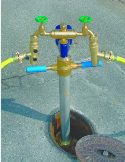
There should be no compromise with respect to drinking water when standpipes are used (Figure: Paguag)
